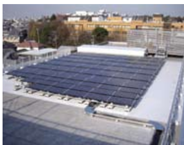
Solar panels installed on the rooftop of the NTT DATA Komaba Training Center
